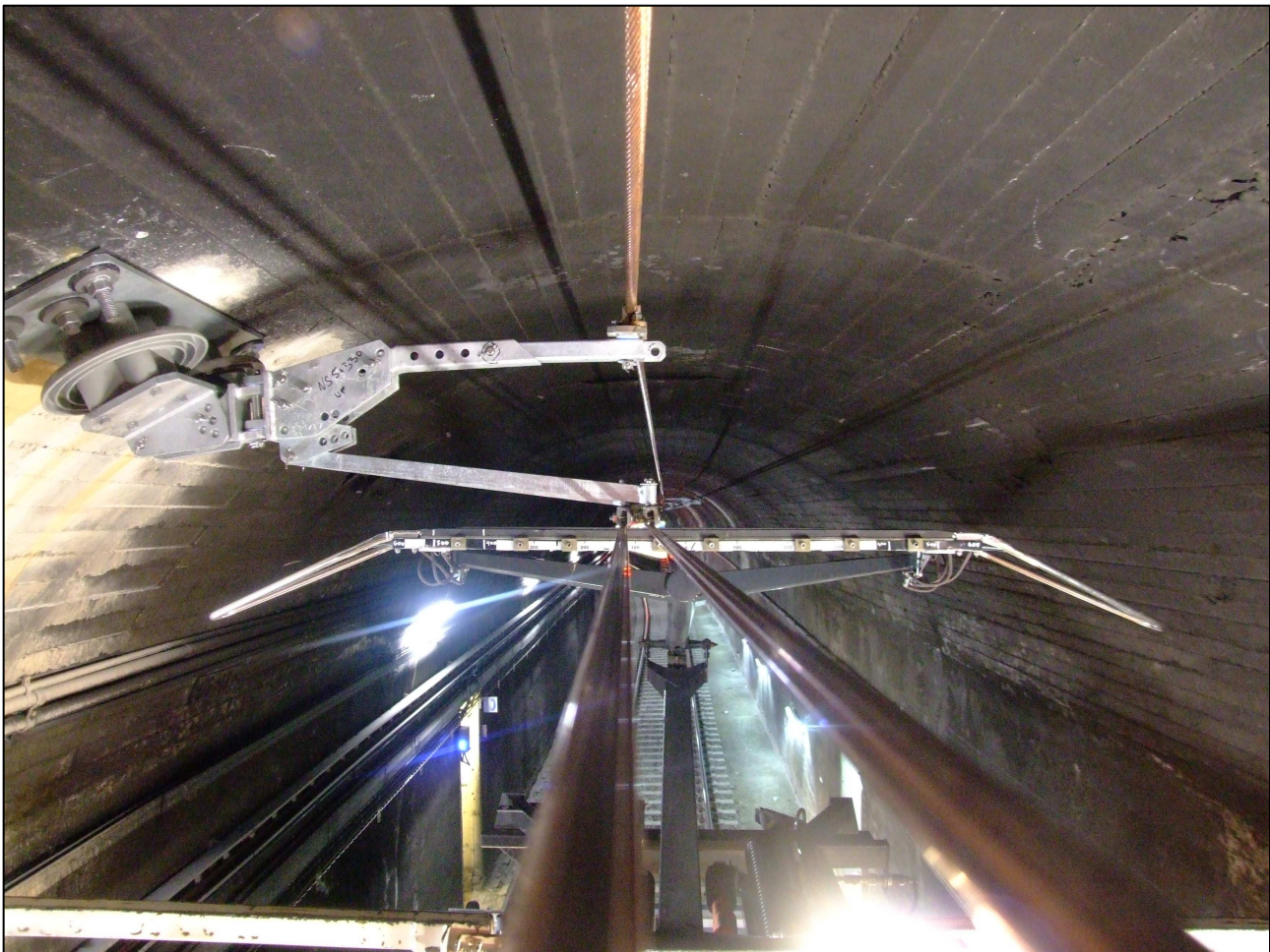
Figure 4 - Installed Mk-3 Tunnel Cantilever at North Sydney (Up Shore Track)
